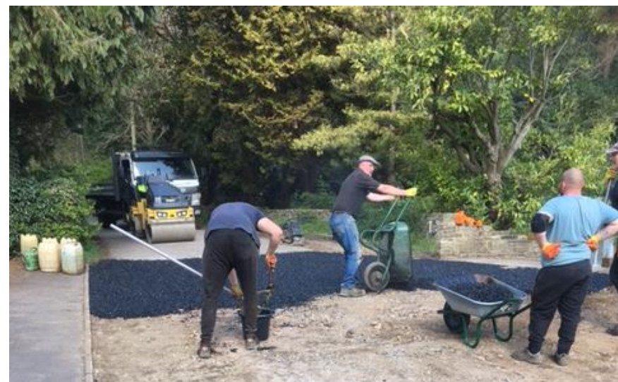
A325 end surfacing
